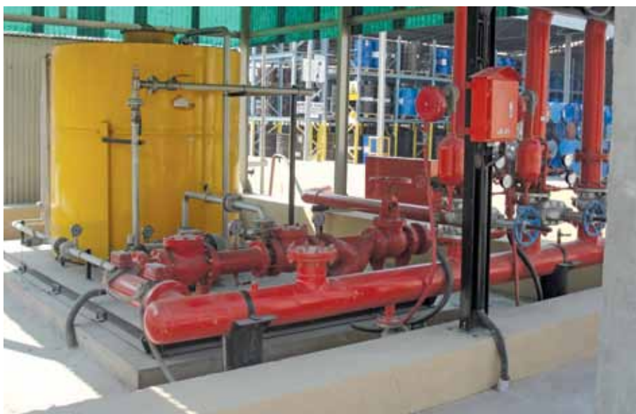
Automatic foam based sprinkler system
